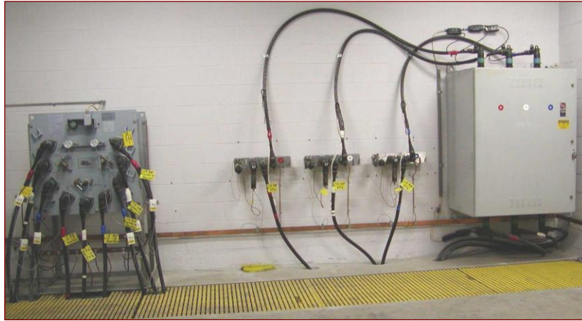
Figure 3-6, Indoor Switching Vault
