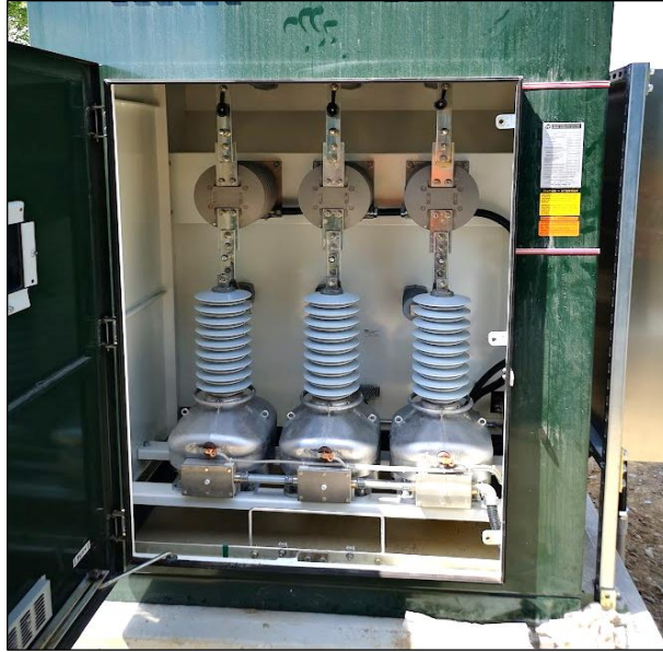
Figure 3-7, Typical Primary Metering Unit
