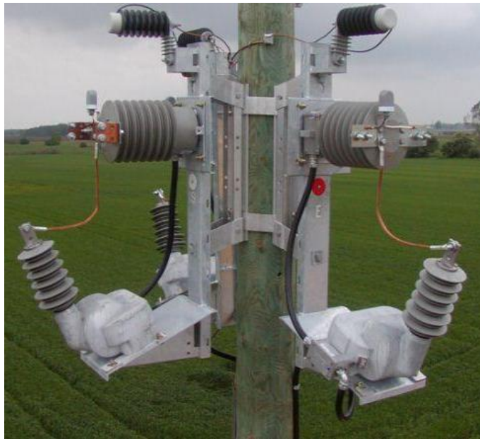
Figure 6-1, Typical Primary Metering Unit
